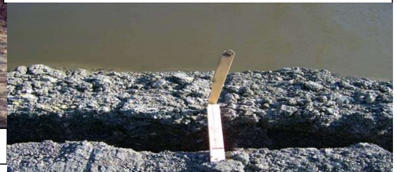
Monitoring of a levee crack.
