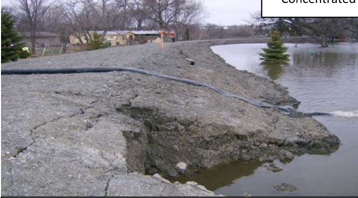
Scour from pump discharge hose.
