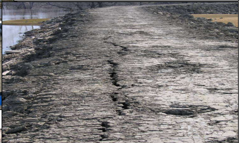
Formation of cracks along the levee.
