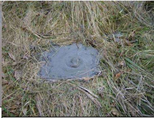
Concentrated seepage boil at levee toe.
