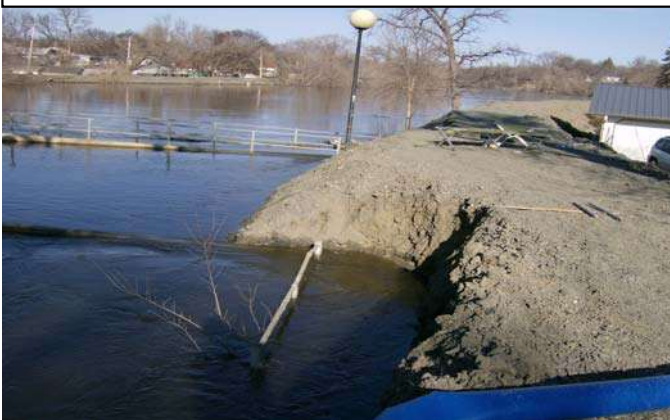
Scour and erosion of levee from river turbulence.
