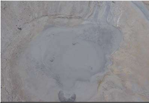
'Dirty' seepage carrying soil particles.
